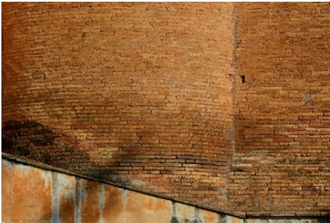
Figure 3. Visible signs of rising damp on a masonry wall in a lateral chapel of San Pietro in Vincoli, Rome. Source: Giaccone, Santamaria and Corradi (2020, Fig. 2b).
